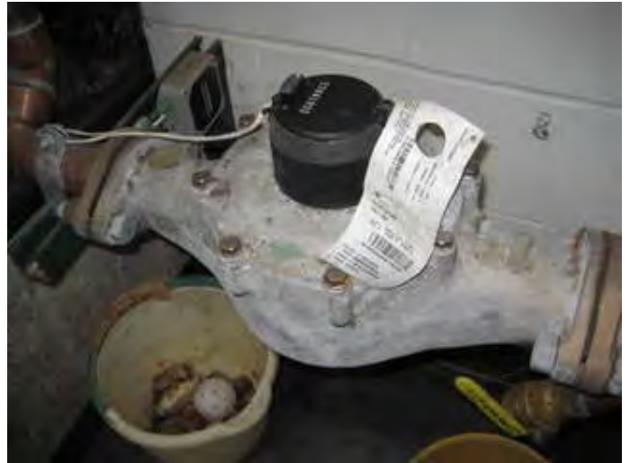
Incoming Domestic Water Meter
