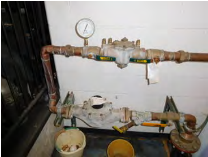
Incoming Domestic Water Service Backflow Preventer
