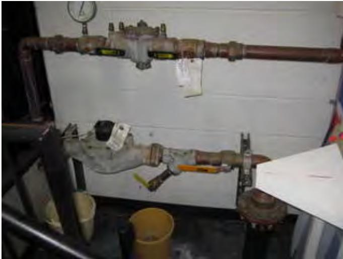
Incoming Domestic Water Service Line
