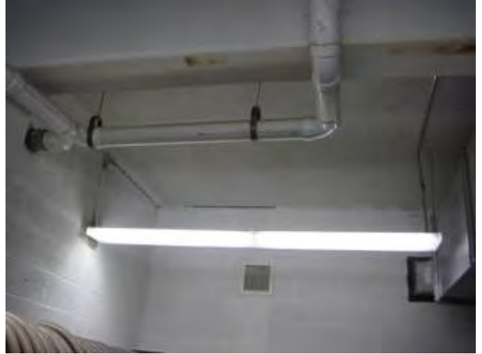
Sanitary Waste Piping
