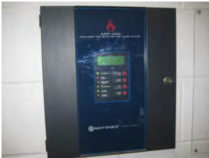
Fire Alarm System Control Panel
