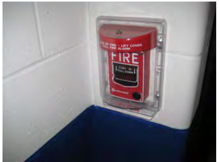
2002 Addition Fire Alarm System Manual Pull Station
