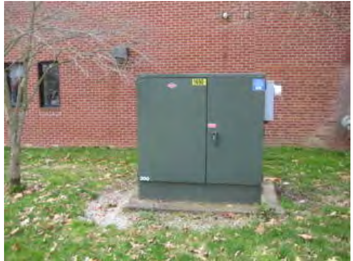
Pad Mounted Transformer
