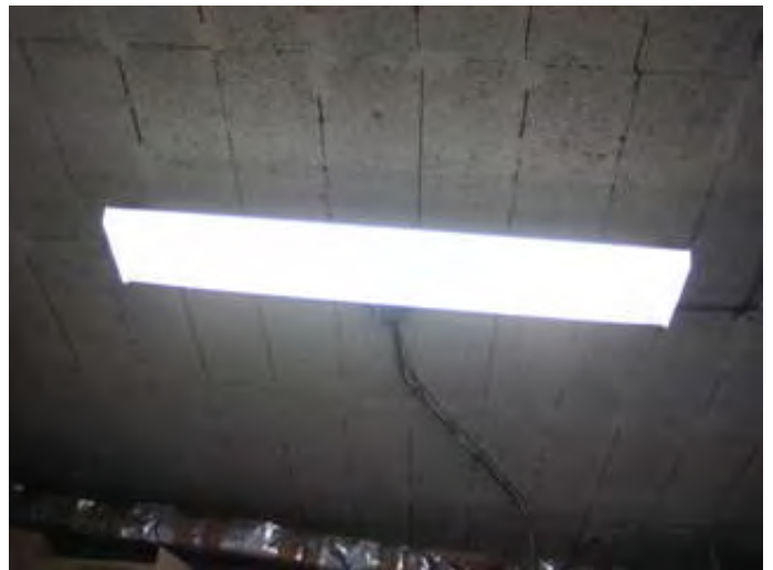
Service Area Fluorescent Light Fixture
