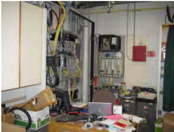
IT System Data Rack
