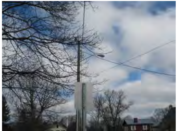
Pole Mounted HID Exterior Light Fixture
