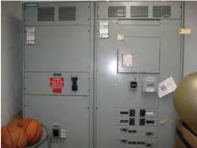
Main Electrical Distribution Panel
