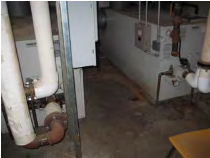
Natural Gas Fired Heated Water Boilers
