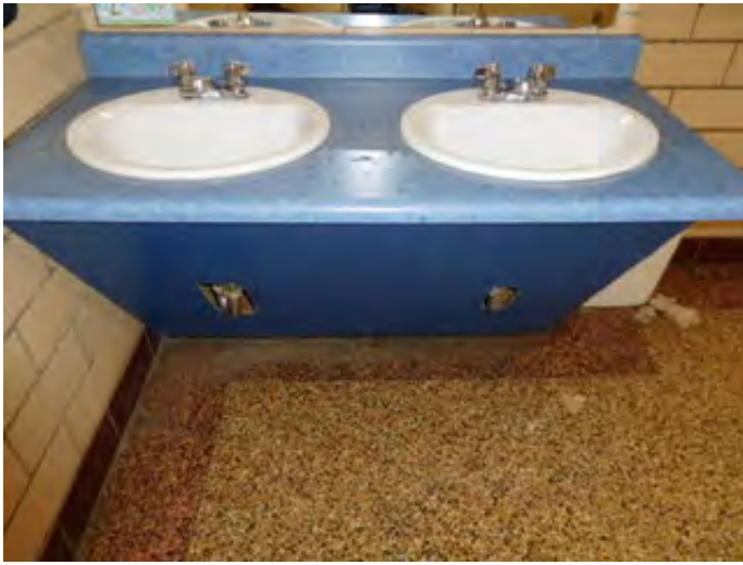
Typical Restroom Lavatory
