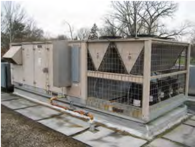
Roof Top Unit
