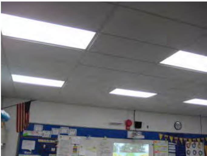
Typical Fluorescent Classroom Light Fixtures
