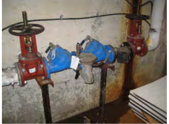
Incoming Domestic Water Service Meter
