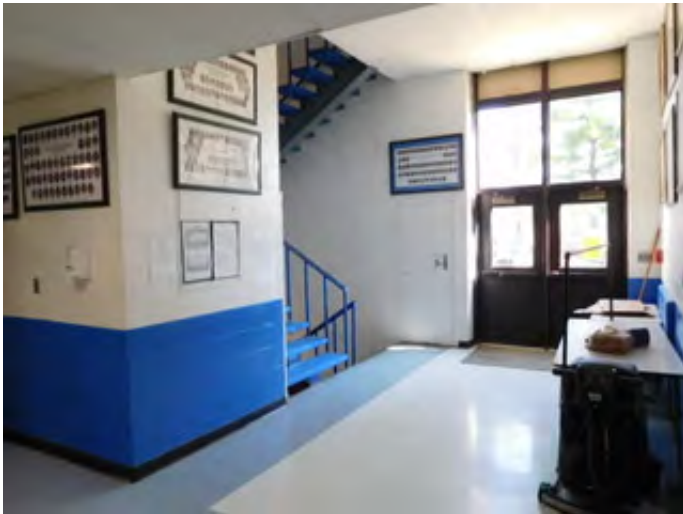
Existing Stair Tower with fire alarm No 2 hour Enclosure
