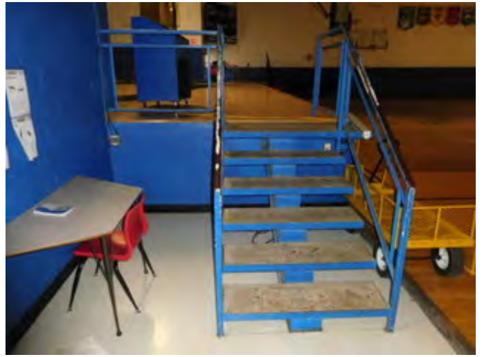
Non-ADA Compliant Stage Access
