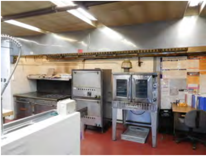
Kitchen Hood & Equipment
