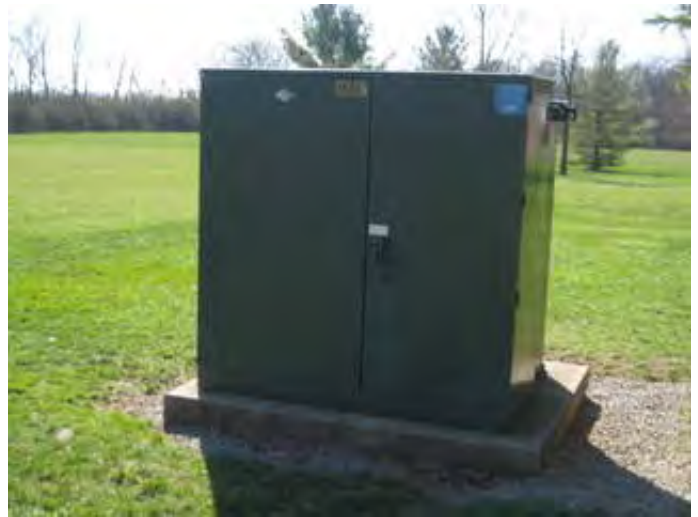
Pad Mounted Transformer
