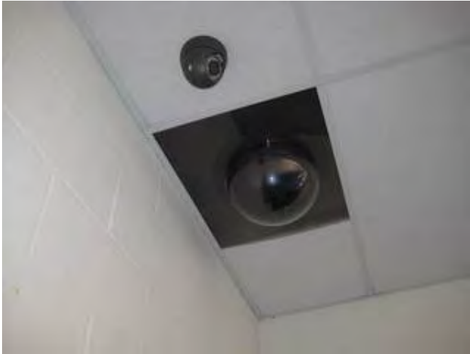
Security System CCTV Camera
