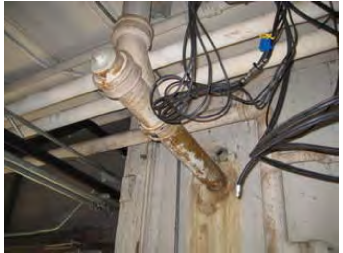
Sanitary Waste Piping
