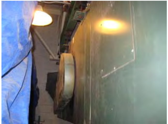
Service Area Incandescent Light Fixture
