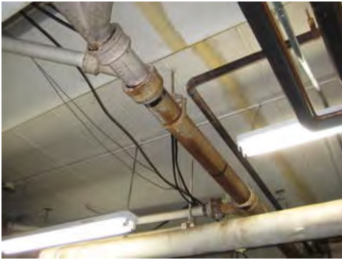
Sanitary Waste Piping
