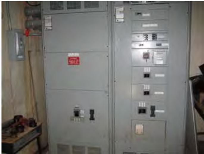
Main Electrical Distribution Panel
