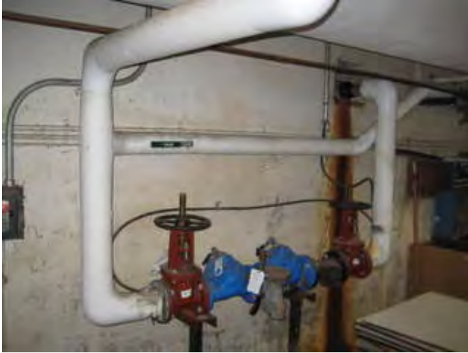
Incoming Domestic Water Service Line
