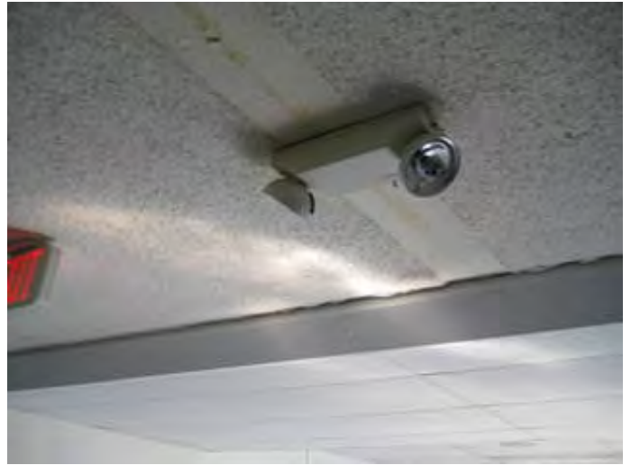
Emergency Egress Light Fixture
