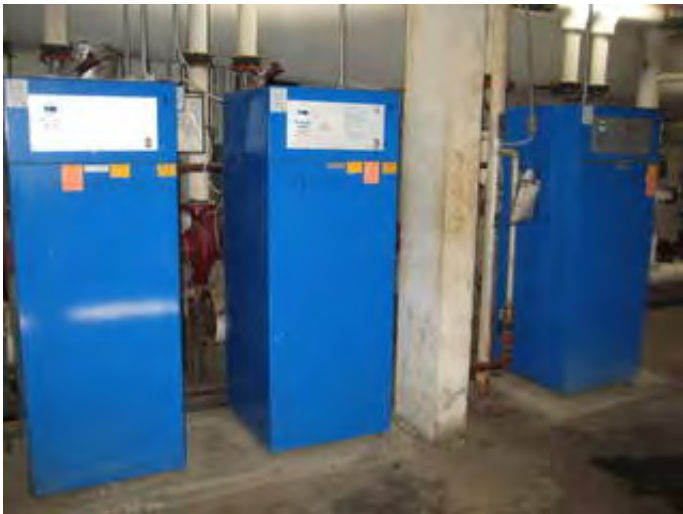
Natural Gas Fired Heated Water Boilers
