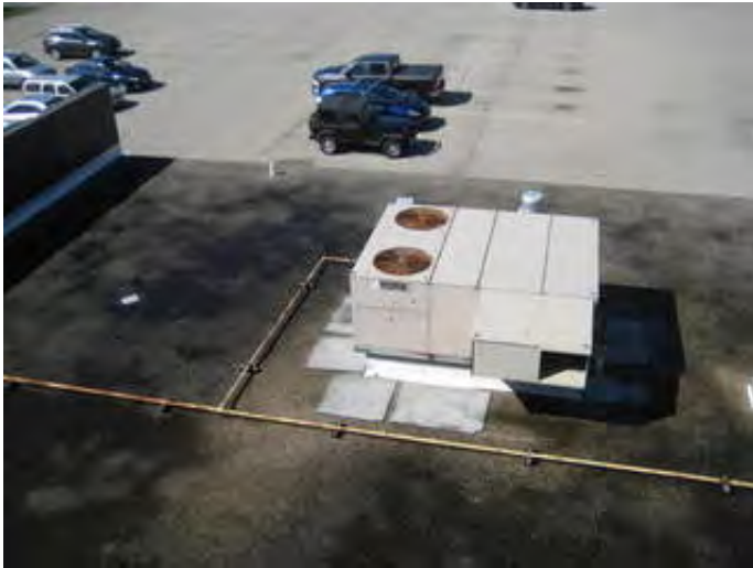
Roof Top Unit
