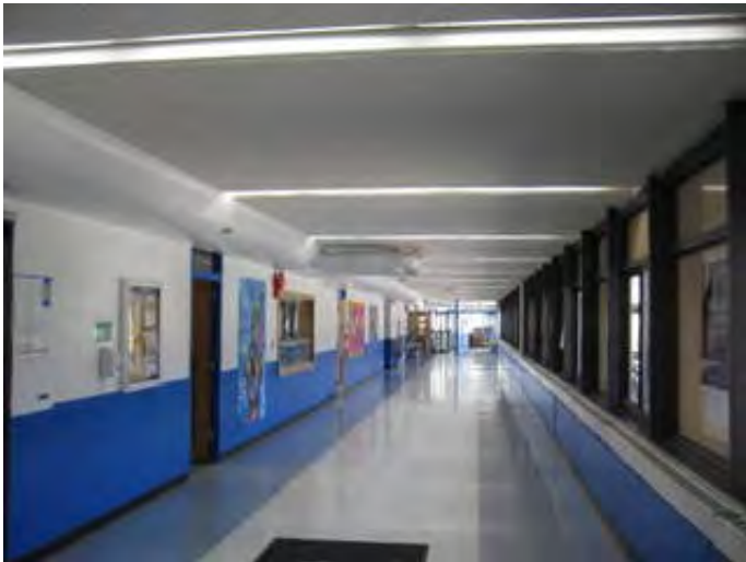
Typical Corridor Fluorescent Light Fixtures
