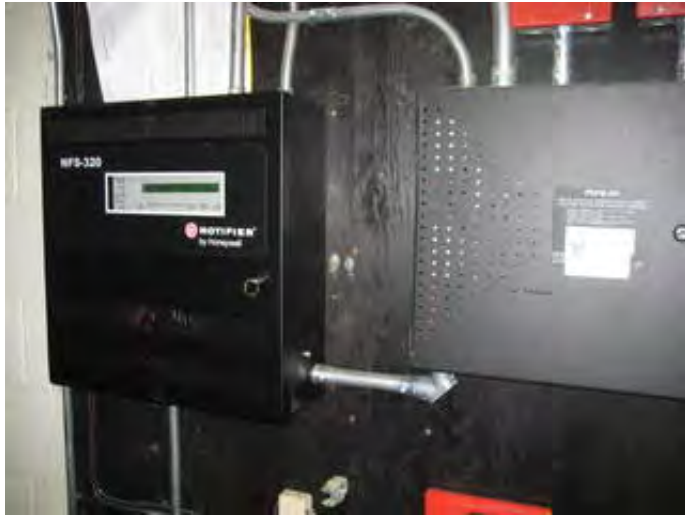
Fire Alarm System Control Panel
