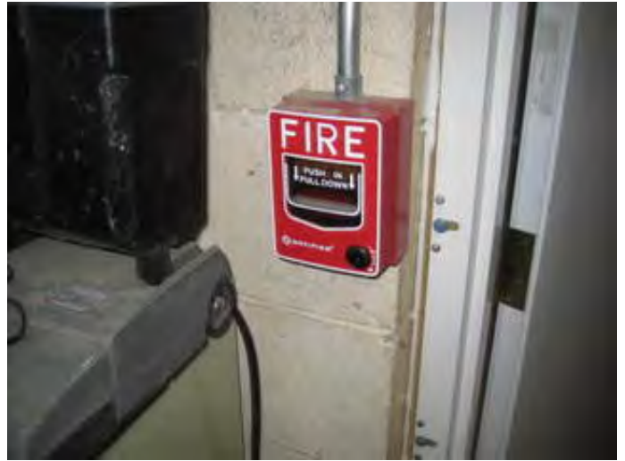
Fire Alarm System Manual Pull Station
